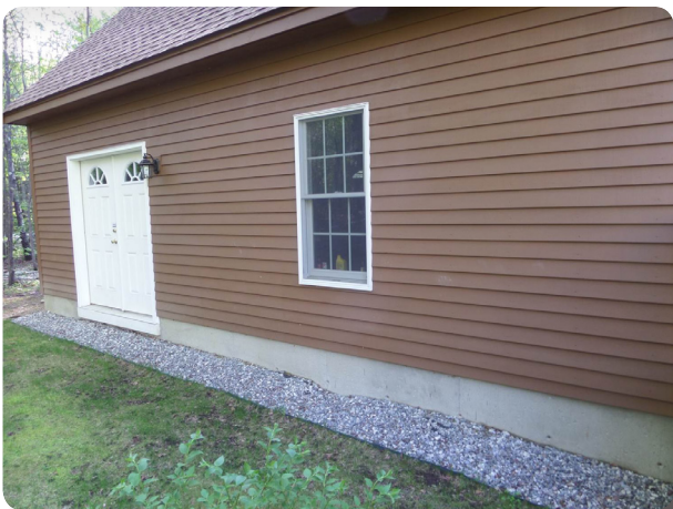
Dripline infiltration trench captures roof runoff.
