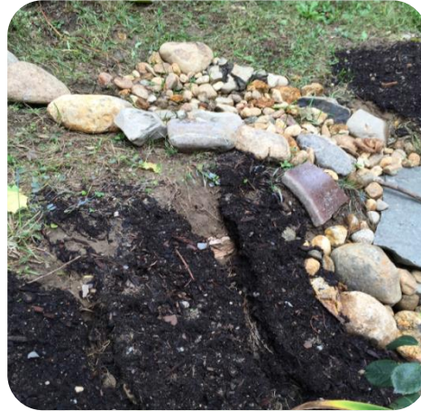
The inlet was widened and stone was added to help guide water into the rain garden.
